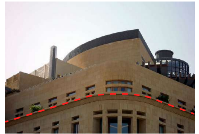
Cornice detail defining the building top expression line; upper roof top shows equipment screening
